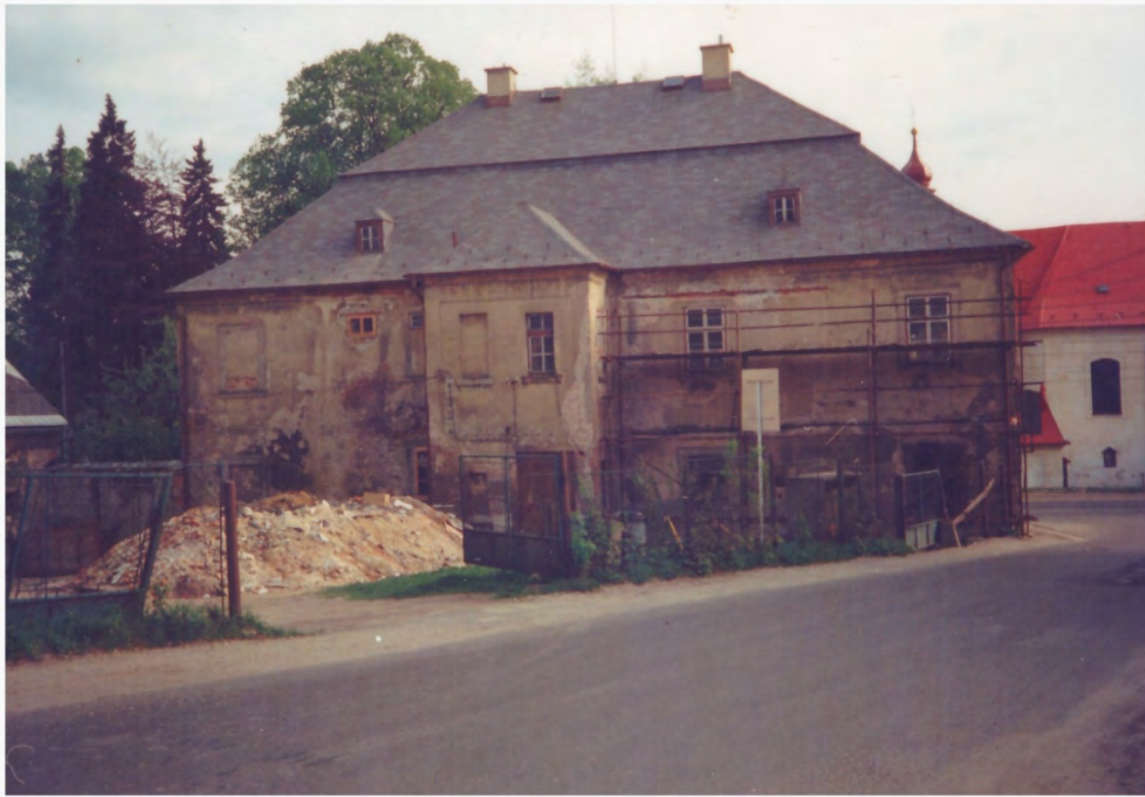
After the Velvet Revolution, the restoration of the rectory begins with the laying of new roofing
